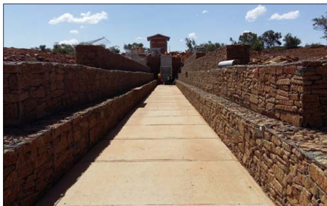
Figure 3: Gabion Zinc coated
